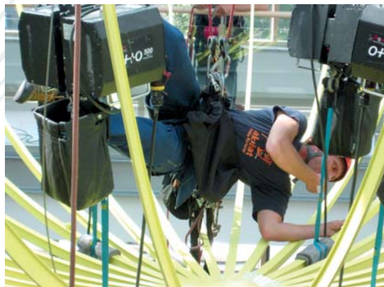
The industrial climbers of Akrobat: they live up to the name of their company as they literally hang upside down to install the Katase sculpture under the glass roof of the DGK.
