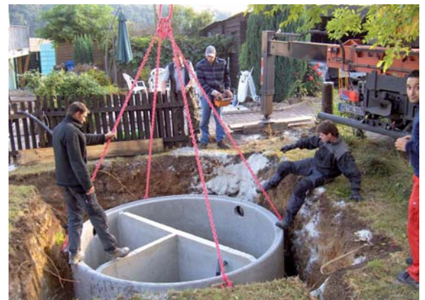
First the planning, then the work: Sciortino builds for himself and his neighbours a complete sewage plant which fulfils all ecological requirements.
