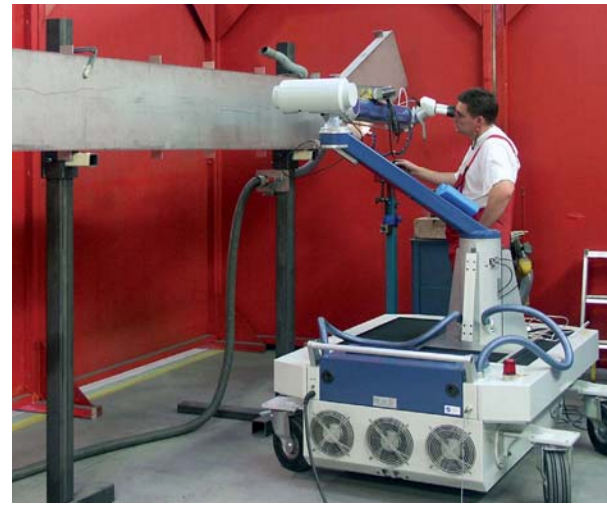
Arnold AG using the Almax: The mobility of this machine allows long welds to be made very precisely up to two meters above floor level.
